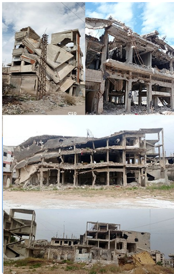
Figure 2 - Completely destroyed buildings that require removal DOI: https://doi.org/10.23670/IRJ.2023.132.35.2
